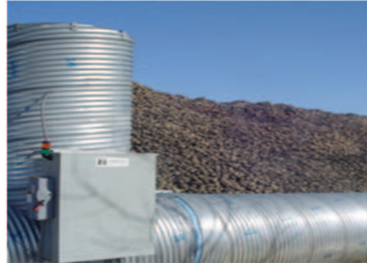
ventilation tower with controls
